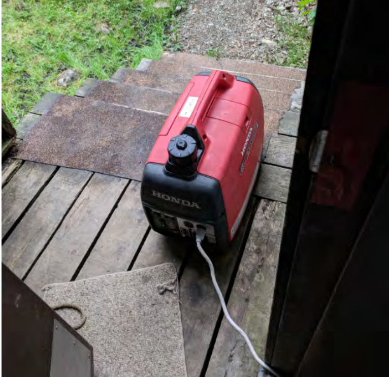
Figure 9: During open hours, library electronics and floor lights are powered by Honda EU 2000i Generator
